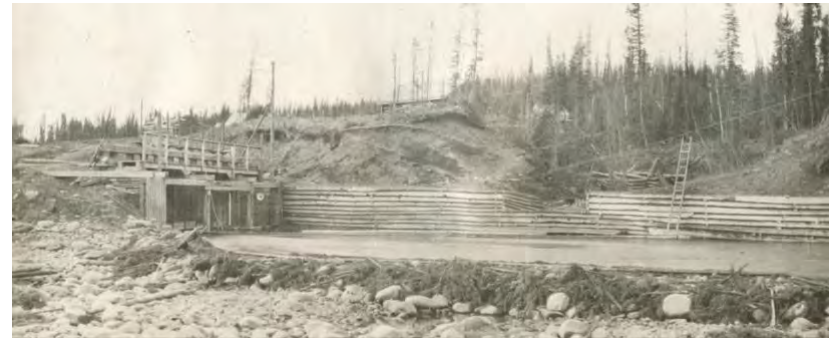
c. 1909-13: North Fork Penstock intake under construction. The Gatehouse has not yet been installed on top of the pressure boxes and penstocks (Yukon Archives).
