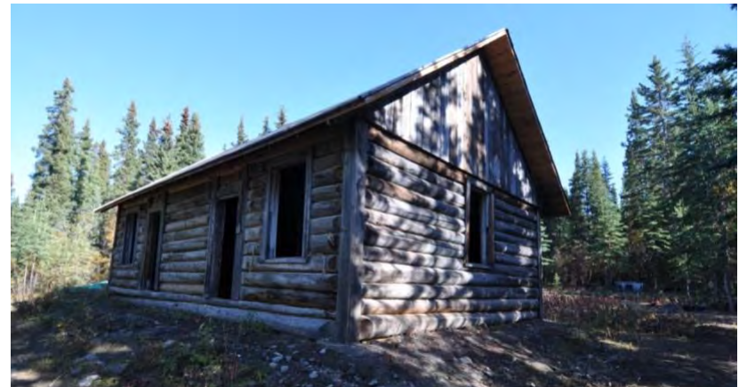
2016: Telegraph Office, south and west elevations after 2015 repairs (Historic Sites Unit, Yukon).
