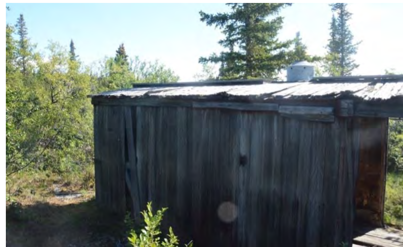
2020: North end of northwest elevation of the Soda Station Boxcar (Historic Sites Unit, Yukon).
