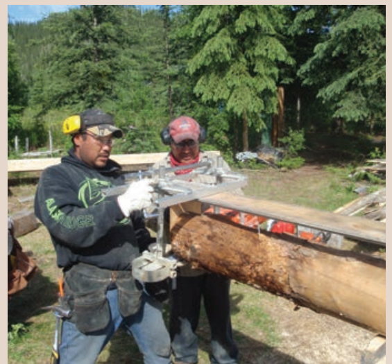
Phillip Bruce, Harvey Kassi milling logs, west side job site. Rampart House. 2016.
