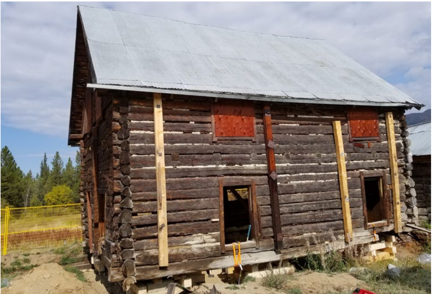
A separated section in the process of being leveled, straightened and raised to a convenient working height.
