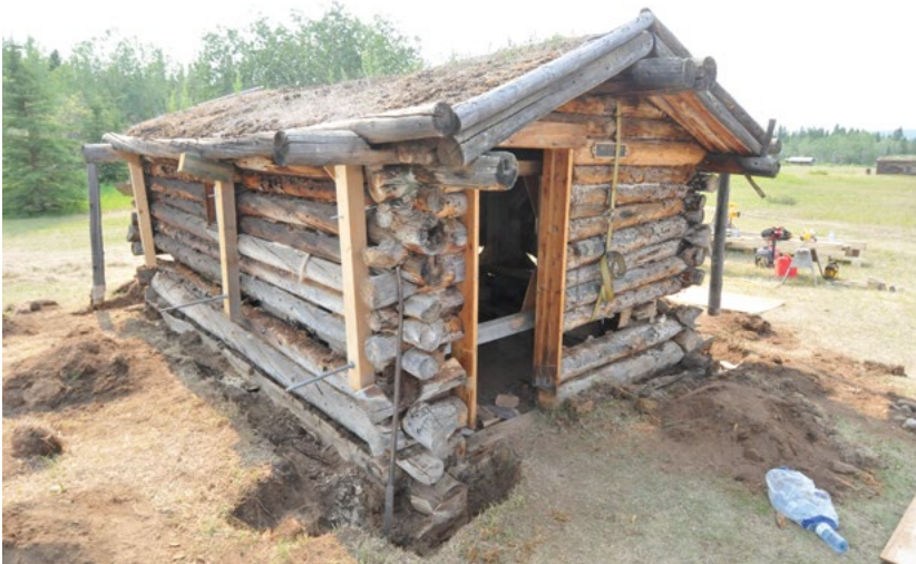
▲ Separation of cabin walls to allow for replacement of lower sill logs. June 2024
