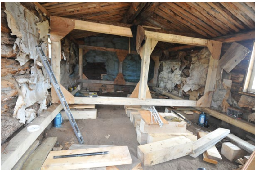
▲ Construction of internal frame to stabilize cabin for lifting. Interior of Tommy McGinty Cabin. June 2024
