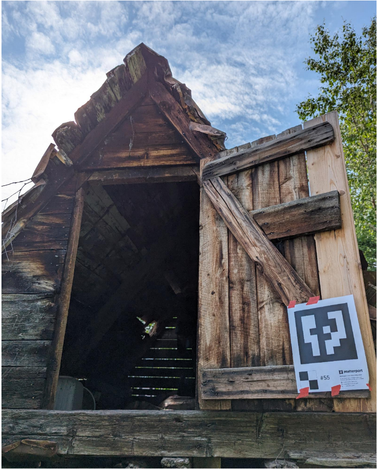
TYP. CONDITION ON EAST ELEV. 10 CURRENT CONDITION (2024) AH107
